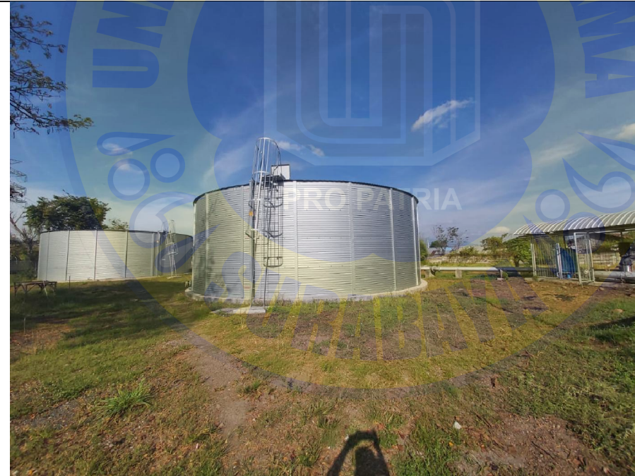
Ground Reservoir Milik PT AB Jatim unit PIER
