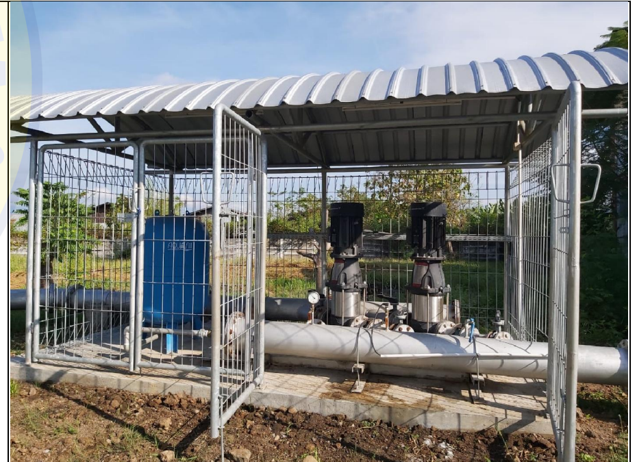
Pompa Sentrifugal jenis VSD ( Variable Speed Drive ) PT AB Jatim
