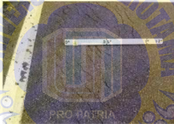
Gambar 2.17 Patah Slip ( Slippage Cracking )
