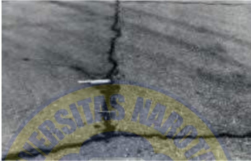
Gambar 2.8 Retak Sambung ( Joint Reflection Cracking )
