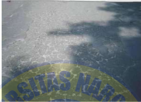
Gambar 2.19 Pelepasan Butir ( Weathering/Raveling )
