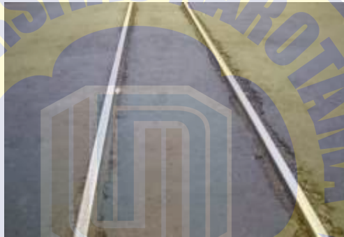
Gambar 2.14 Rusak Perpotongan Rel ( Railroad Crossing )
