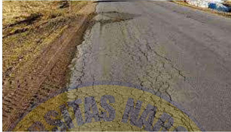
Gambar 2.7 Retak piggir ( Edge Cracking )
