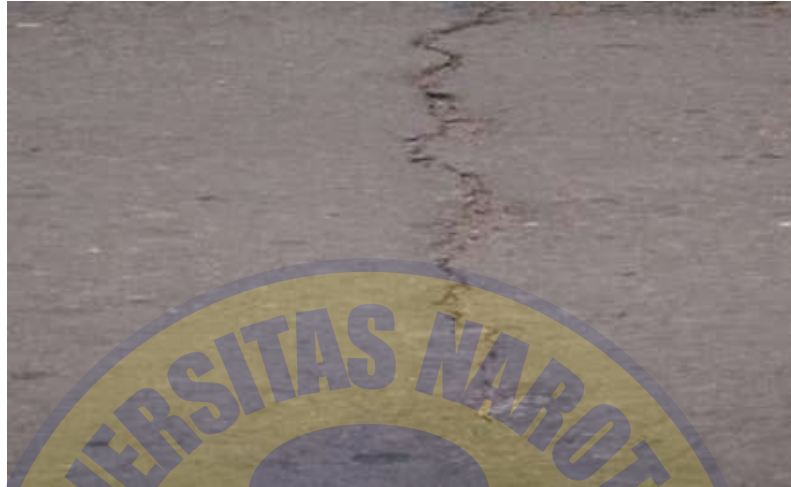
Gambar 2.9 Retak Sambung ( Joint Reflection Cracking )
