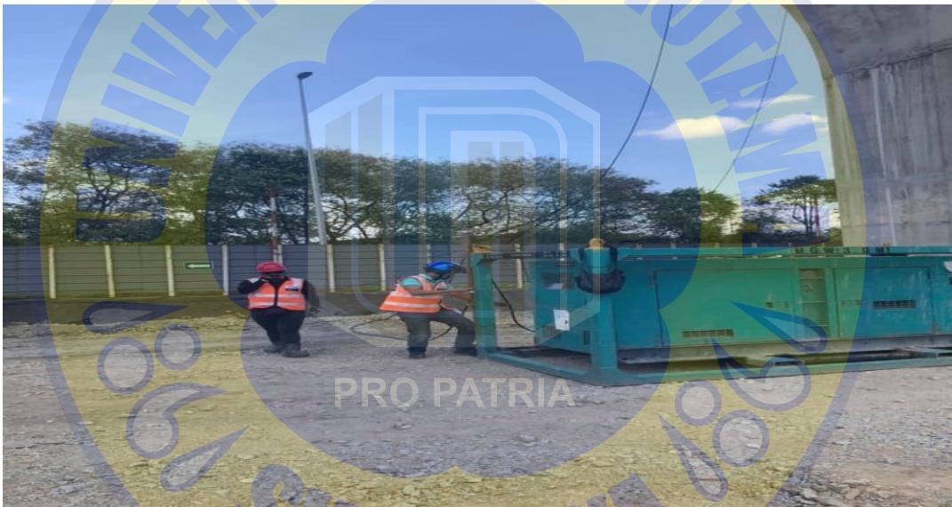
Figure 4.1 Workers are Working on How is the Waste System Throw to Container Safety
