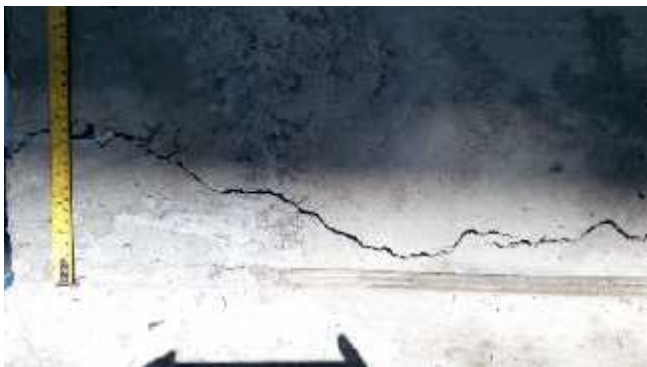
Fig. 9 Crack Wall Foundation
